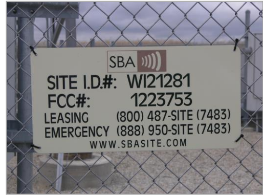
Exhibit 8-9. An example of appropriate tower signage placed on the security fence
