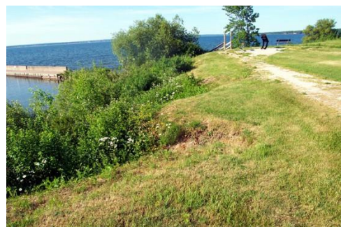
Top of Bluff in the Central Coastal Area of Washburn next to the Marina showing Signs of Erosion (SWB, Inc.)
