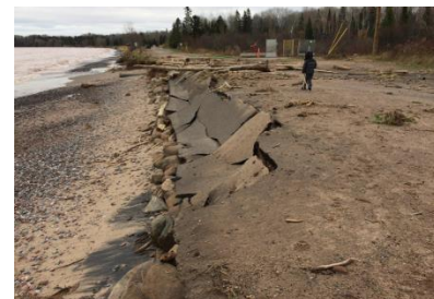
Erosion of road along Lake Superior in Herbster, WI: Photo by Dennis Fawver (October 2017)
