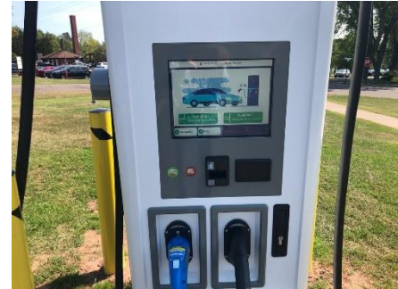
Electric Vehicle Charging Station (Cheq Bay Renewables)
